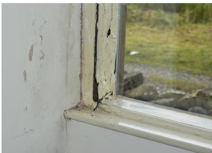
Showing the serious decay on the west window
