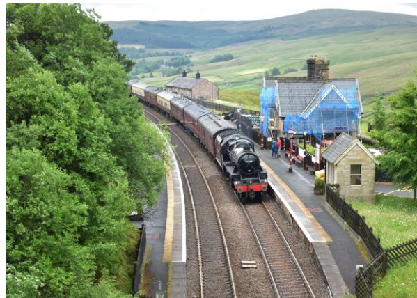
'Black 5' 44392 passes Dent on 1 st July 2023 with the building still shrouded in blue netting
