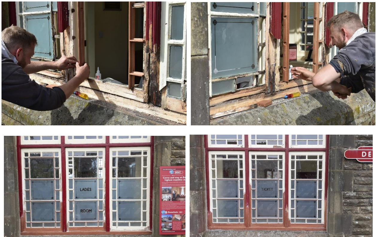
Philip Middleton carefully re-assembling the decayed elements of the windows and the completed work before decoration (June 2022)
