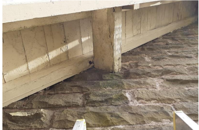
A decayed purlin on the west gable
