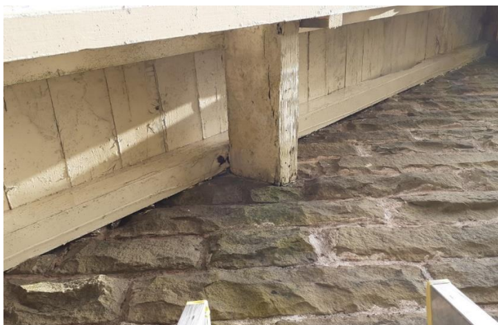
A decayed purlin on the west gable
