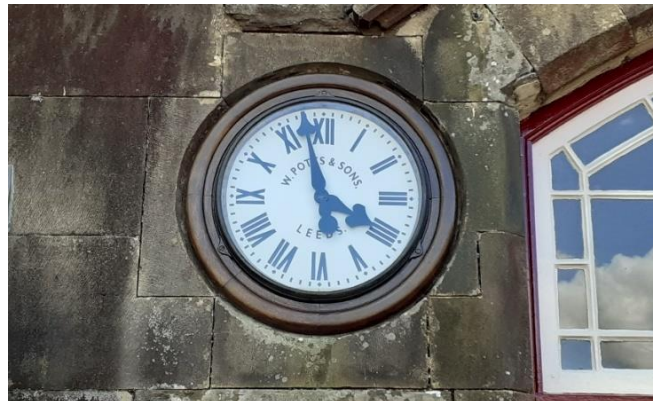
The restored W Potts & Sons station clock now looks the part (September 2022)
