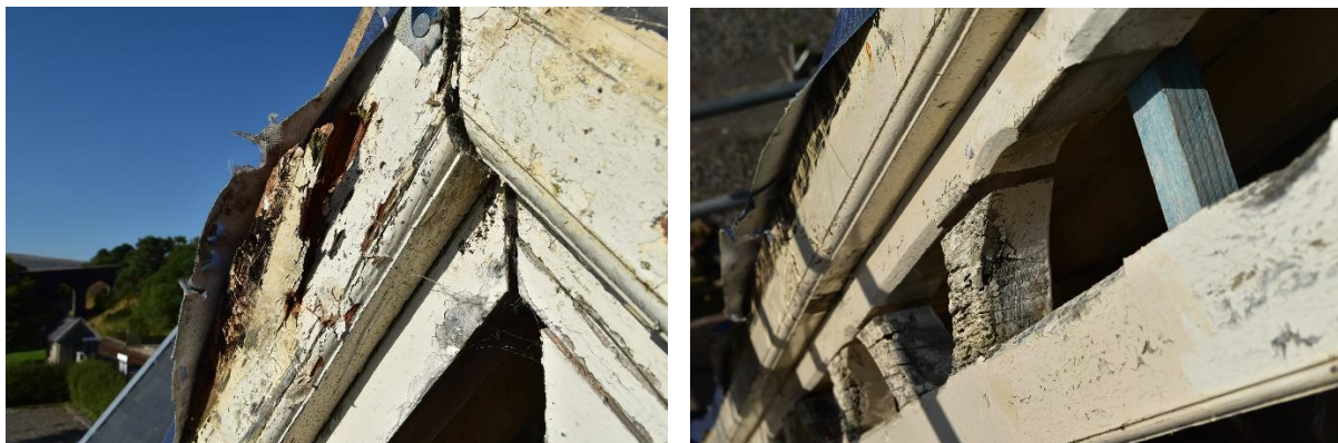
Showing the state of the gable barge boards (2021)
