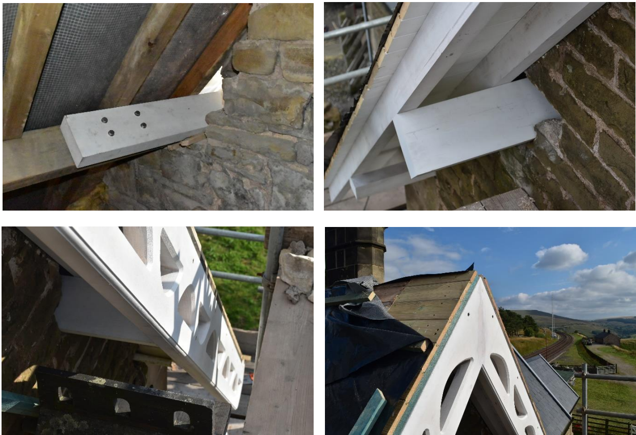
New purlins (showing the bolted connection) and barge board in place (September 2021)
